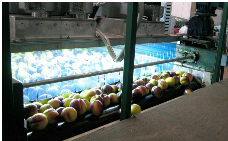
A Light Progress installation in peaches process line
